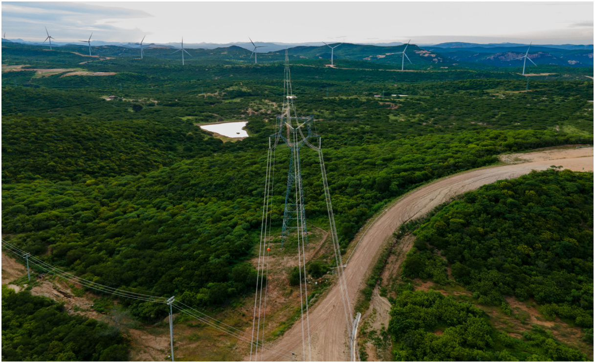
Figure 16 São Paulo–Minas Gerais transmission line
