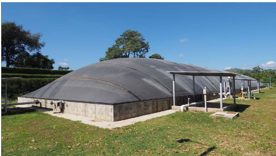
FIGURE 6: Covered lagoon digester
