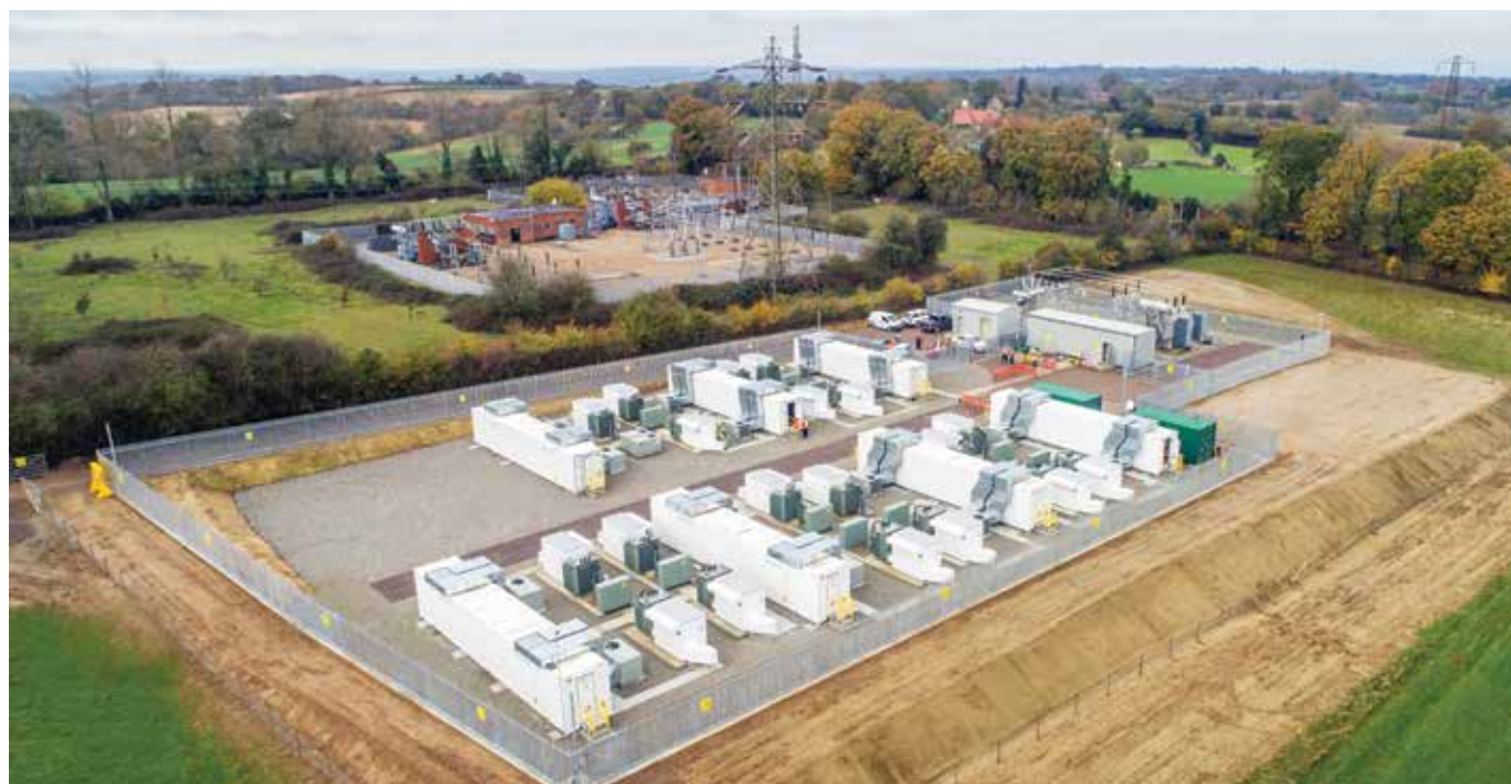
Figure 31: Low Carbon’s Glassenbury project
