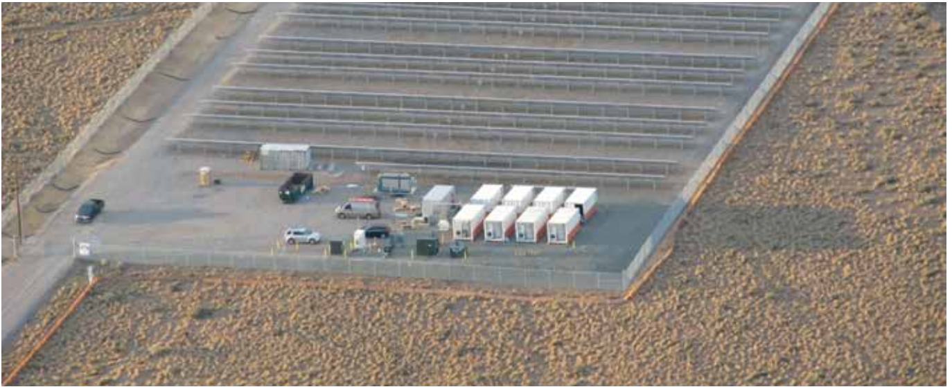
Figure 47: Batteries at the Prosperity energy storage project in New Mexico
