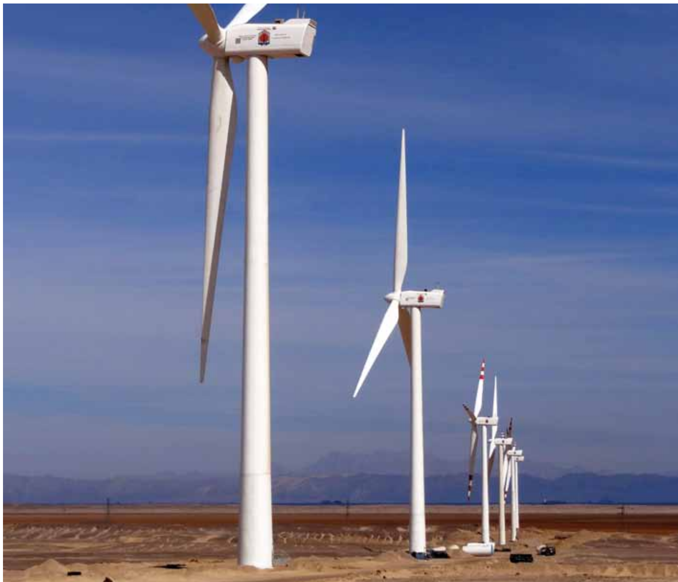
200 MW El Zayt Wind Farm, Egypt Photograph: RCREEE
