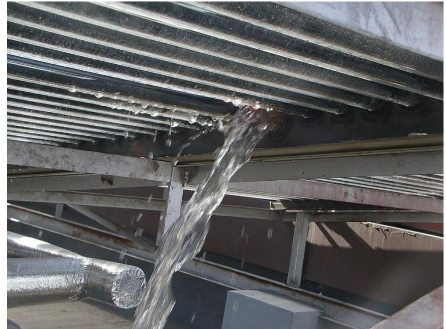
System failure conditions (water leakage)
