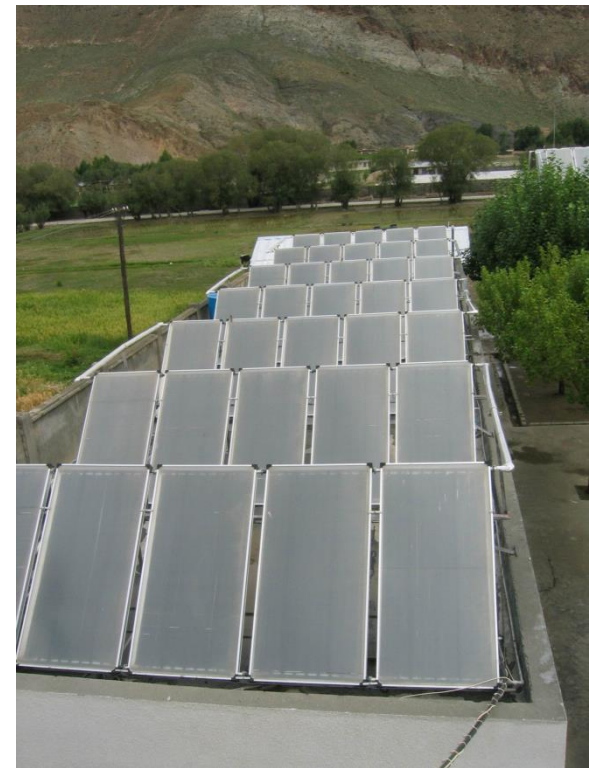
Flat plate collectors in one camp site
