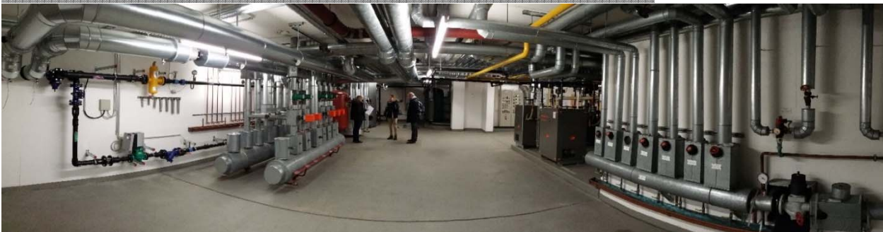
Mine water use for space heating, Germany
