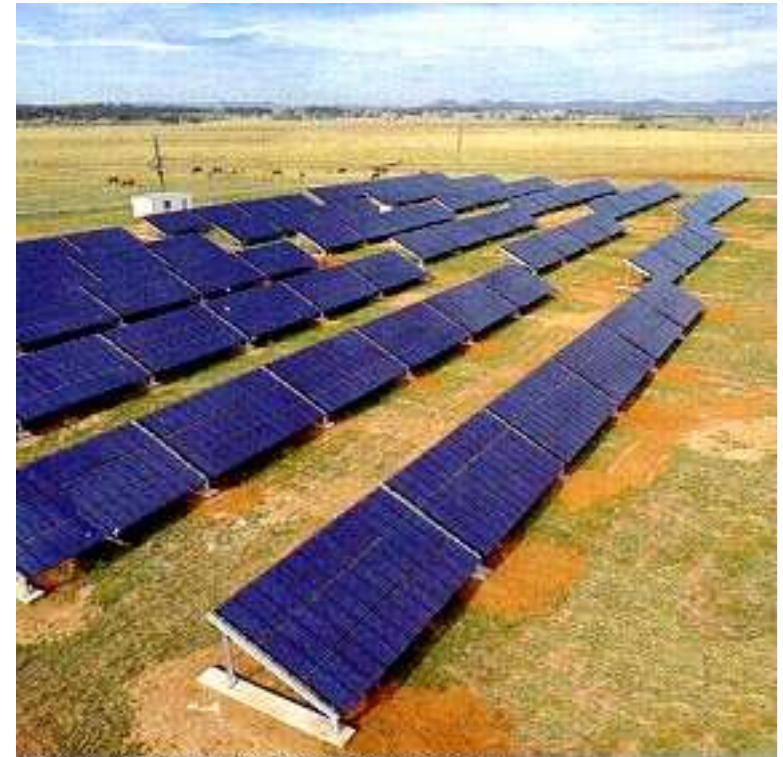
The Singleton photovoltaic solar array
