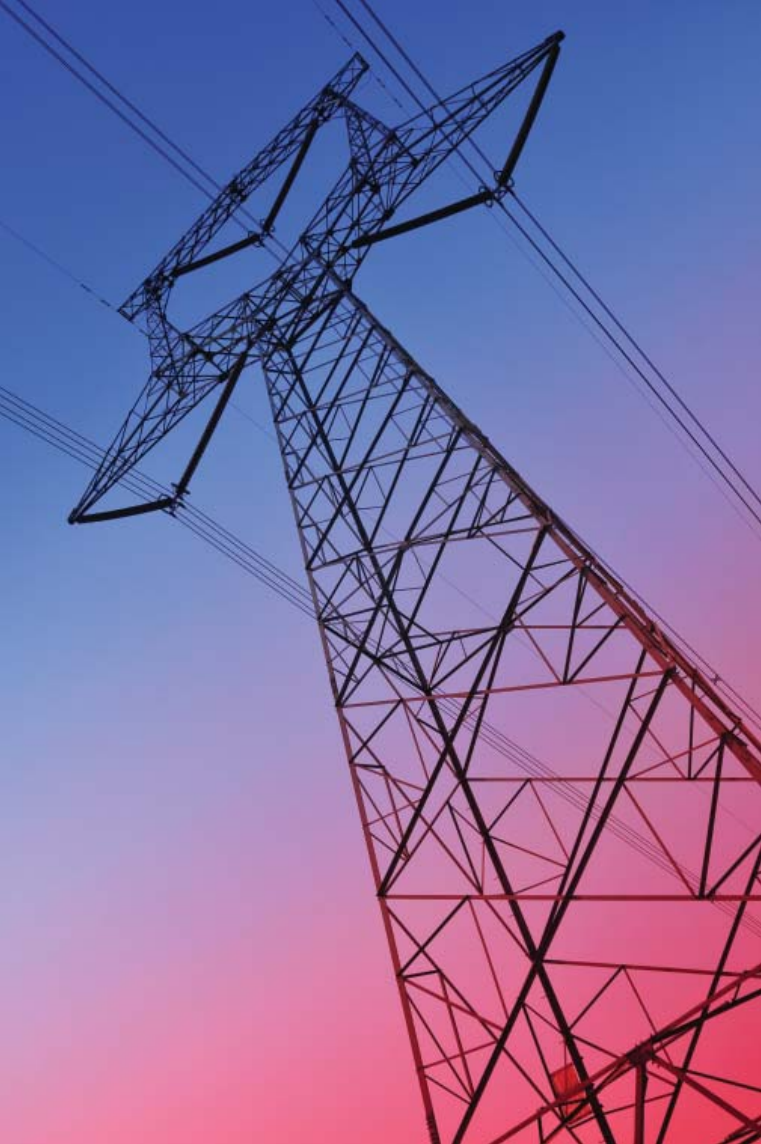
Transmission tower Photo Courtesy: Shutterstock
