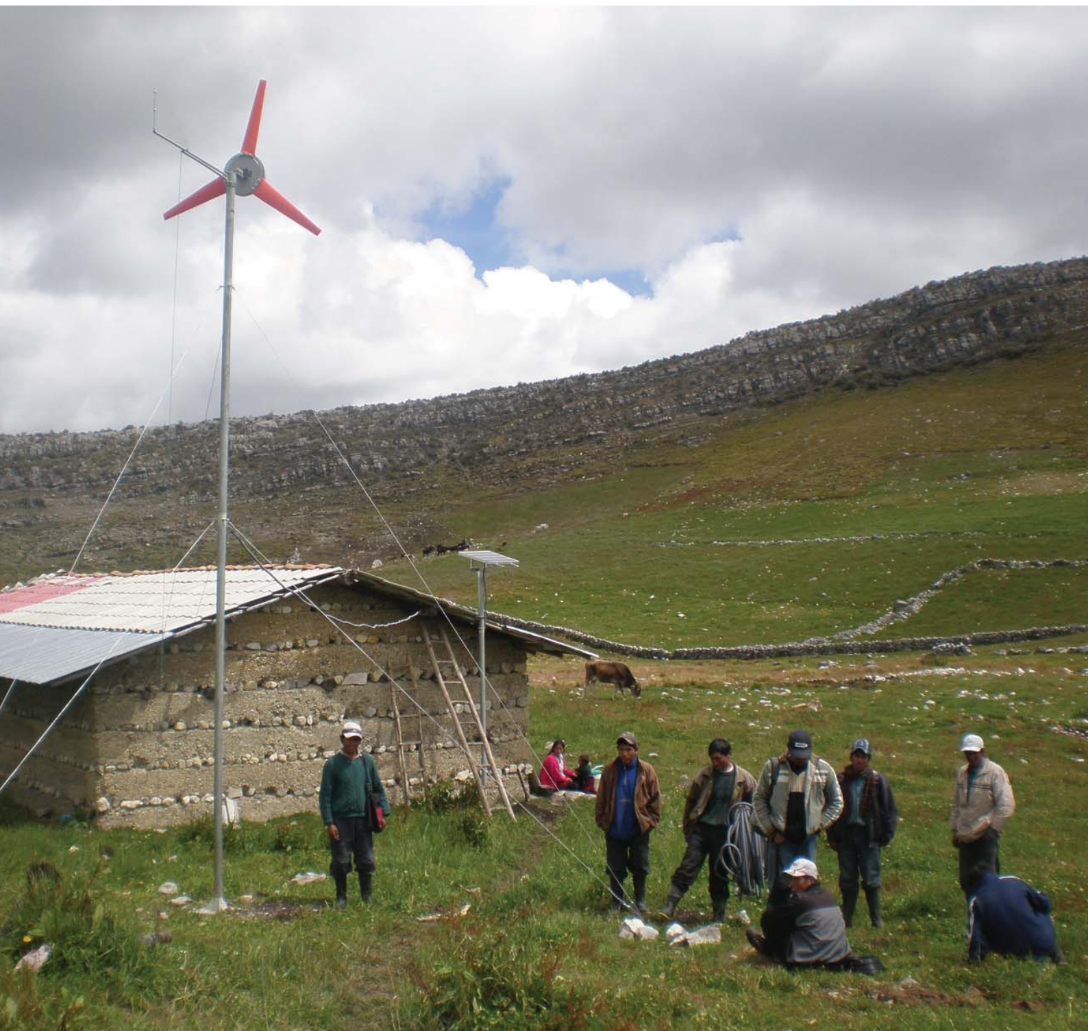
Off grid rural renewable energy system, solar PV and wind Photo Courtesy: MINEM Peru
