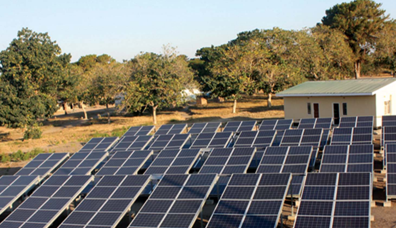
Solar photovoltaic power plant Courtesy: REA
