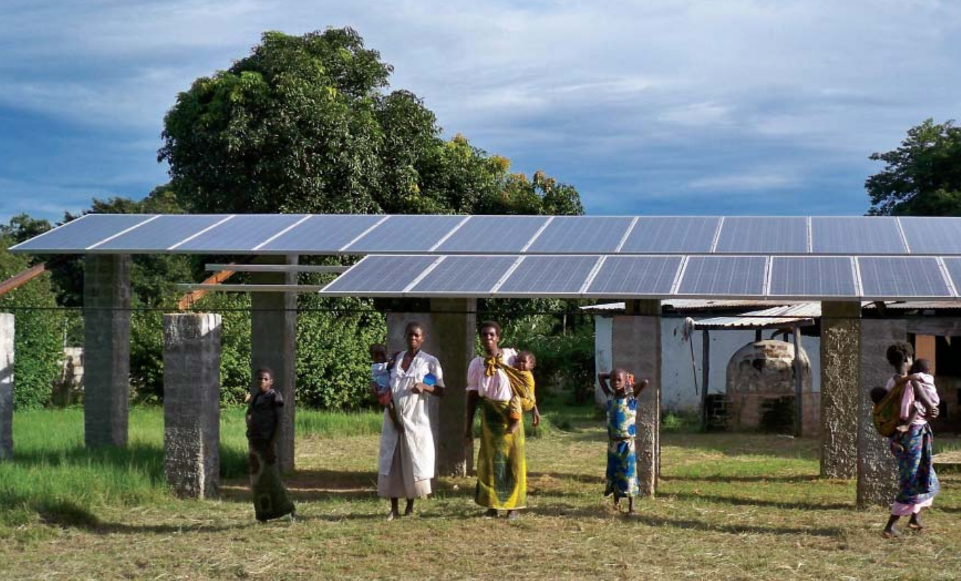
The Chitokoloki Hospital has 24-hour power generated by several banks of solar batteries, a large battery storage area and an inverter. The new system is able to handle almost all the hospital demands Source: www.chitokoloki.com
