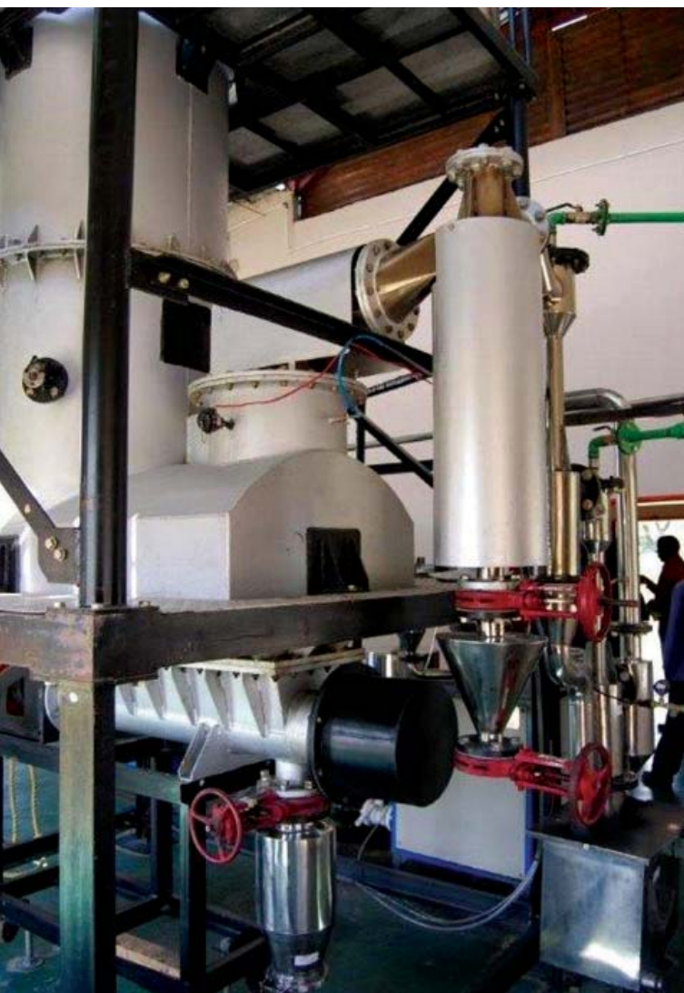
Biomass power generation. Courtesy: REA
