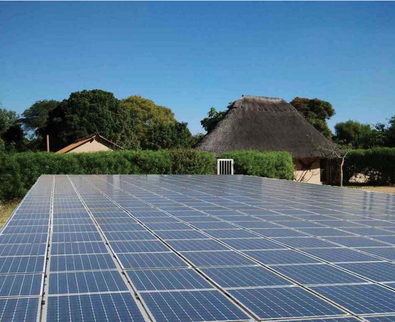
Photovoltaic panels Courtesy: REA
