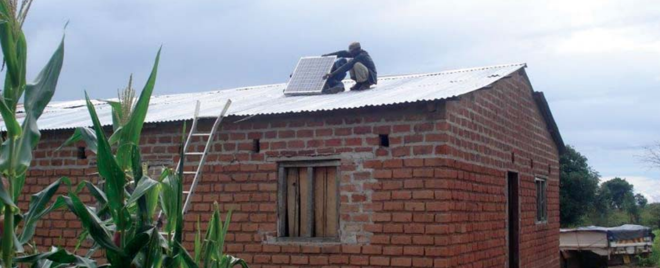
Roof-mounted solar photovoltaic: rural electrification. Courtesy: REA
