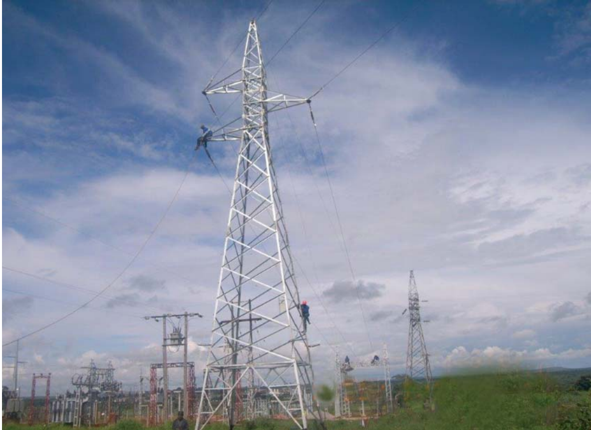
Grid transmission lines in Zambia Source: REA
