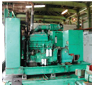
Current Use: Cummins Genset 400 KVA 10-20% CNO in Diesel Fuel Savai EPC Power Station, Samoa, 2005 Source: Gilles Vaitilingom
