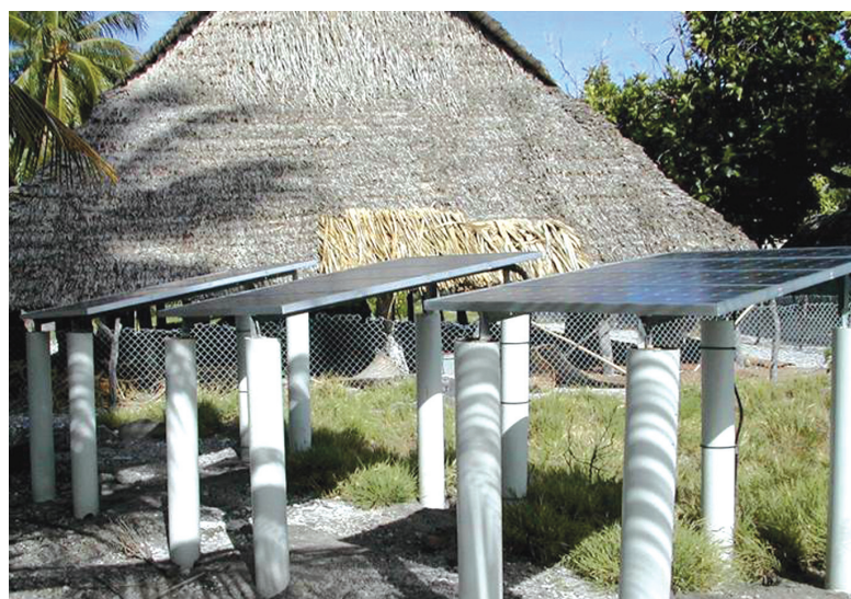
A maneaba solar PV system in North Tarawa
