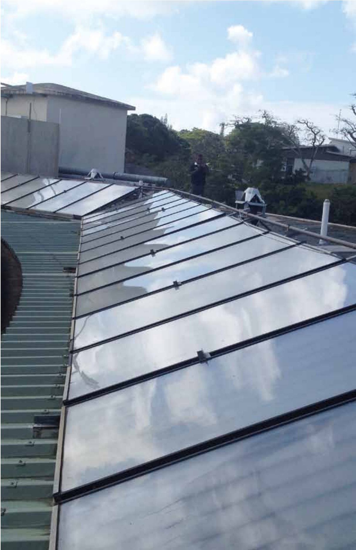
Solar Water Heaters, Grand Hotel Port Vila Photo: H. Wade
