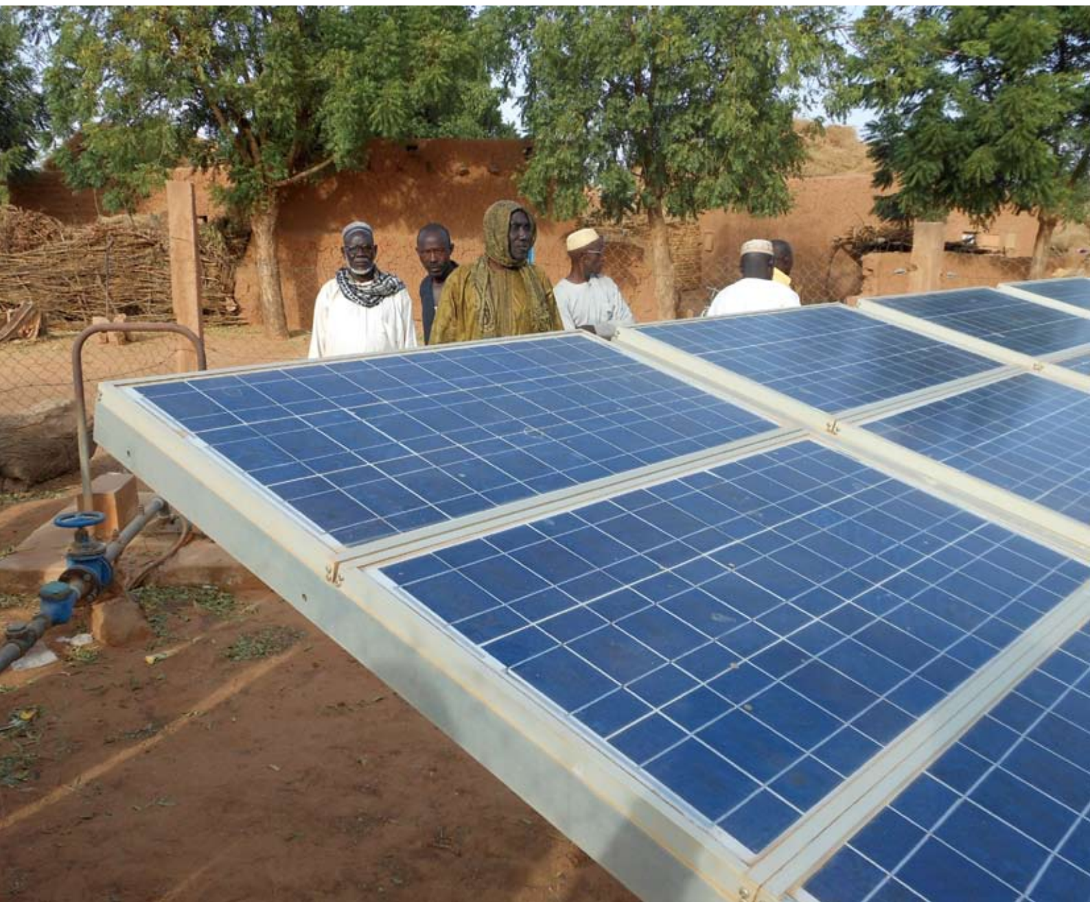
Solar water pumping system in Tondigameye Village, Niger Photo: IRENA/G. Singh
