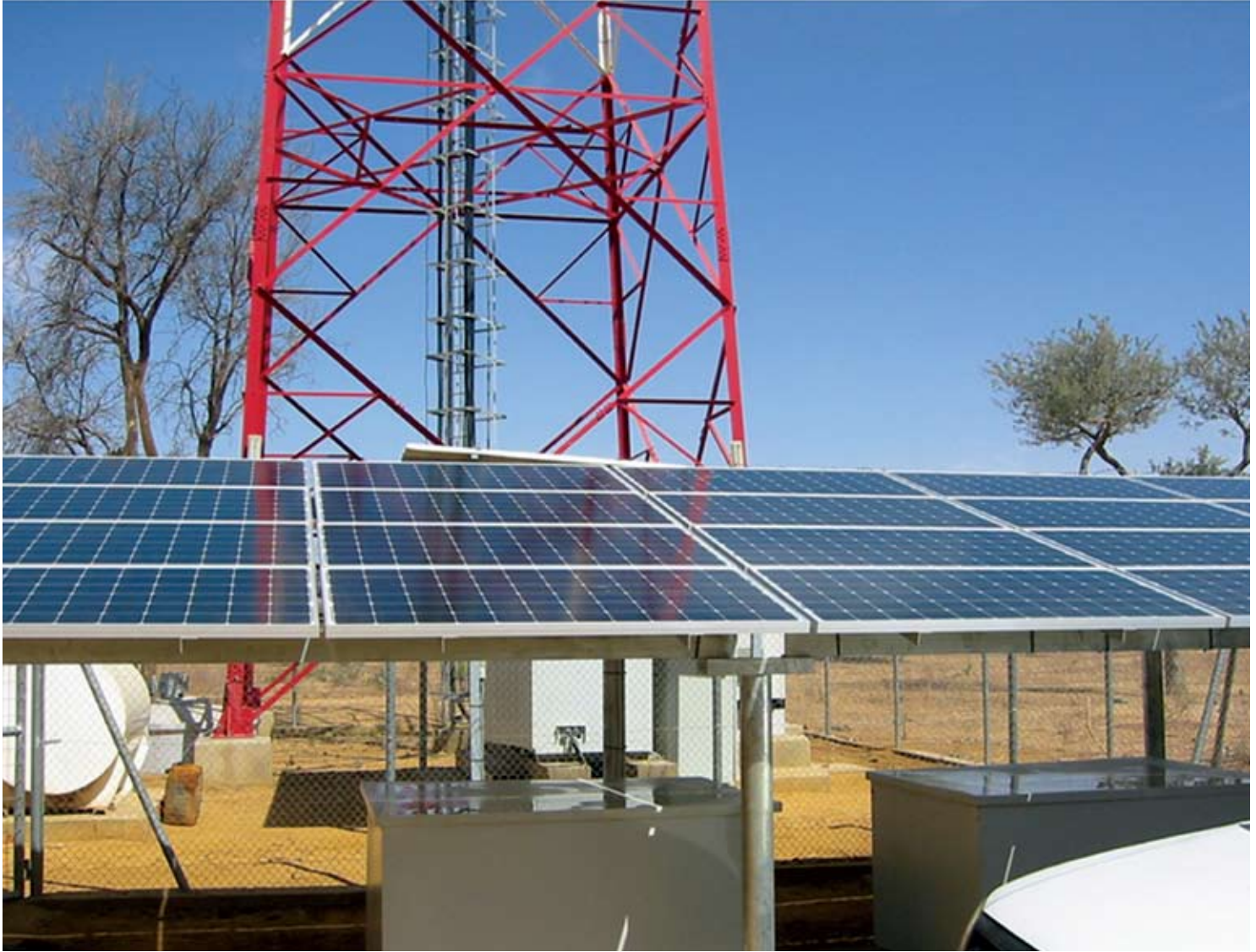
Solar PV system for telecom tower Source: Airtel Niger
