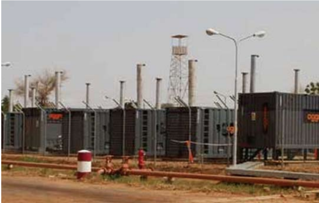
Diesel power plant in Niamey Source: www.nigelec.ne
